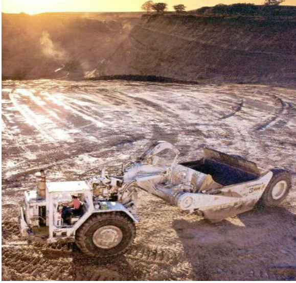
Figure 6: The use of earthmoving scrapers greatly accelerated the rate at which overburden was removed. Source: CONOCO.
